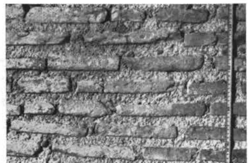
Fig. 89d. S. Martino ai Monti, Roman Hall, brickwork c; south façade of vaulted Hall after rebuilding
